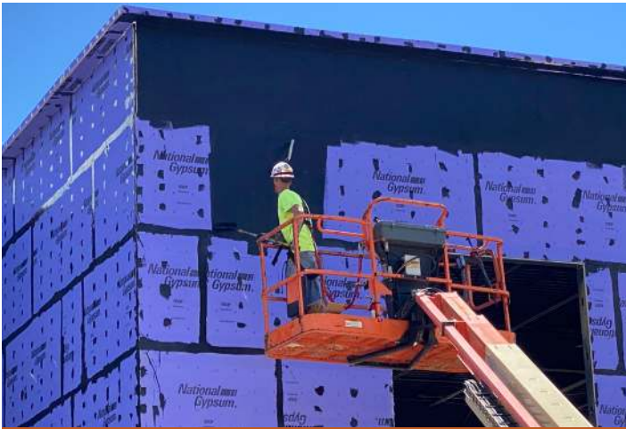
Adhesion testing assesses whether air and water resistive barrier coatings on substrates have sufficient strength to maintain integrity of the building envelope.
